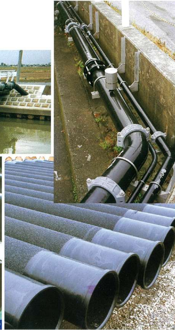
Buried trunk-line gas pipeline (high frequency induction bend + external F type)
